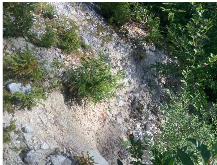
Fill slope instability
